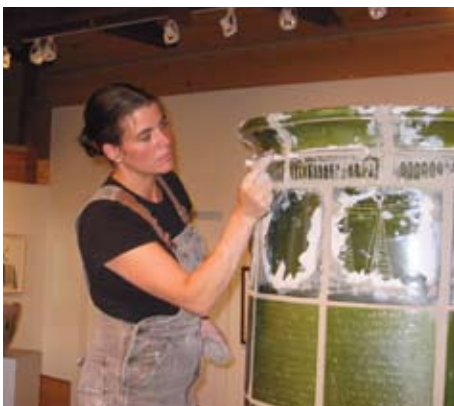
As the rows of kacheln are set, Steinhäuser removes wooden spacers and finishes the outside mortar joints. Excess mortar is removed with a sponge.
